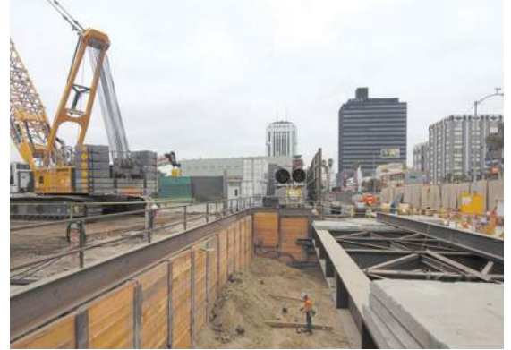
Coordination of underground utilities is critical to safely and efficiently operate Metro service.
