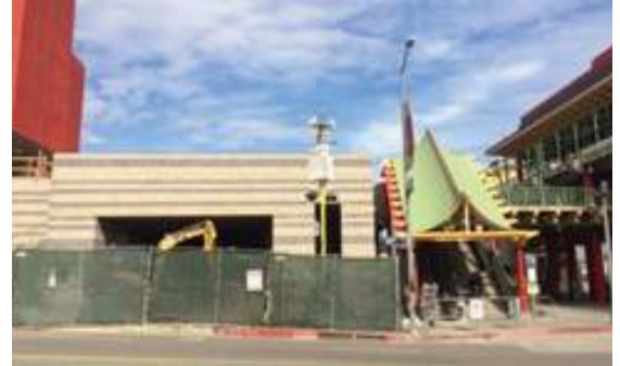
Sidewalk access is blocked for a construction project, forcing pedestrians into the street or to use less direct paths to the Metro facility.
