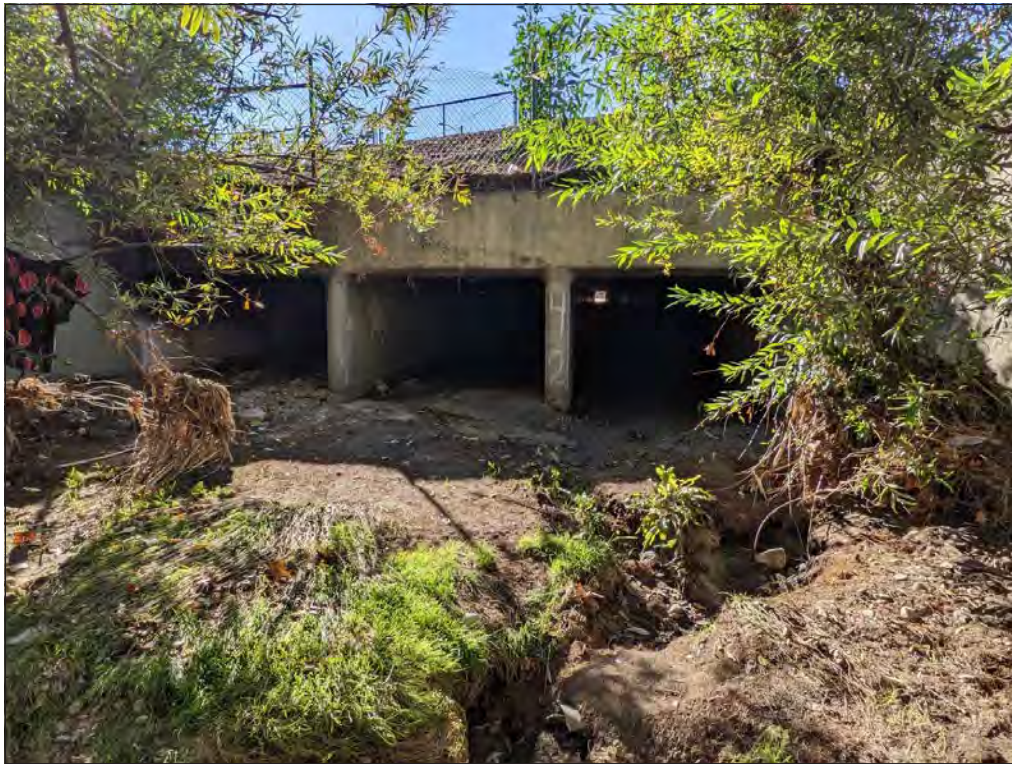
Photo 1: View of the upstream portion of Honby Channel, facing south. Sediment accumulation and erosional issues can be seen.
