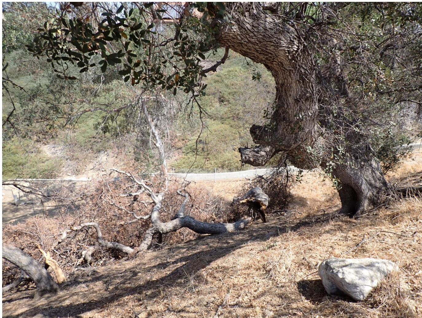
Facing north – illustrating Trees #78's limb failures. Cavities are present in the trunk and scaffolds, and this tree has an active bee hive in the main trunk.
