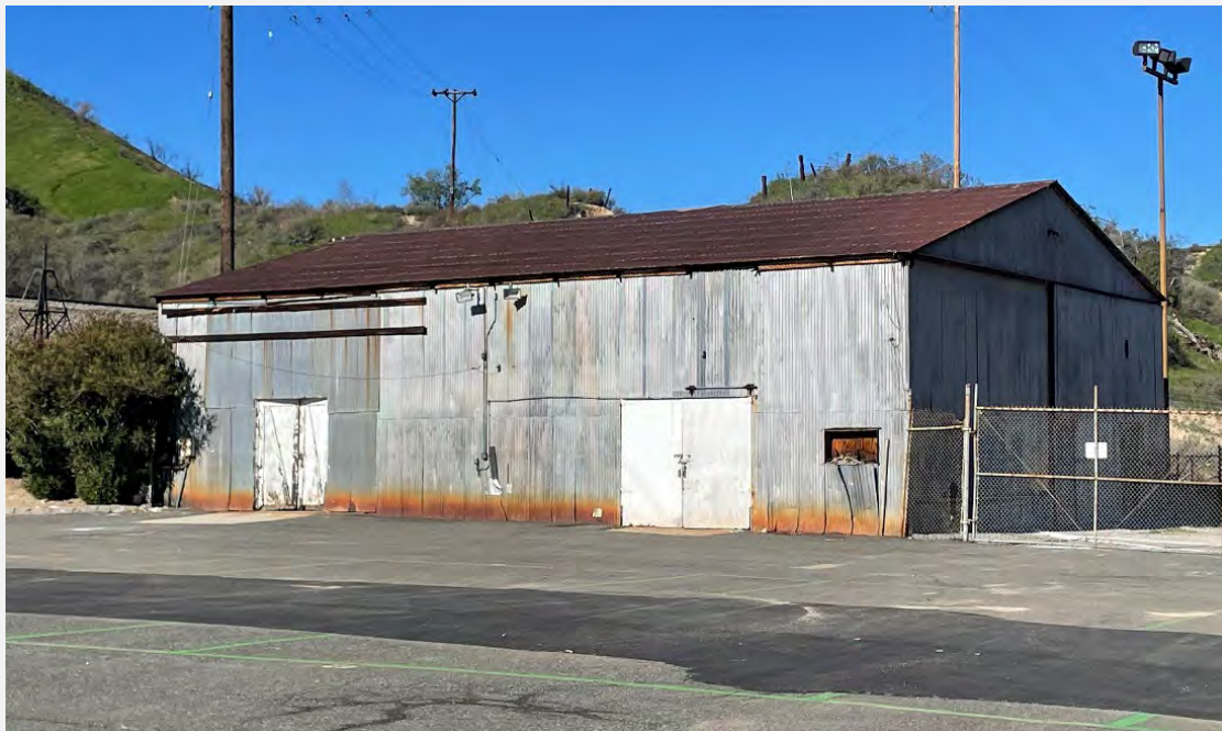
Figure 12. Overview of the Warehouse (3) primary (southeast) and side elevation. View looking west (IMG_3169).
