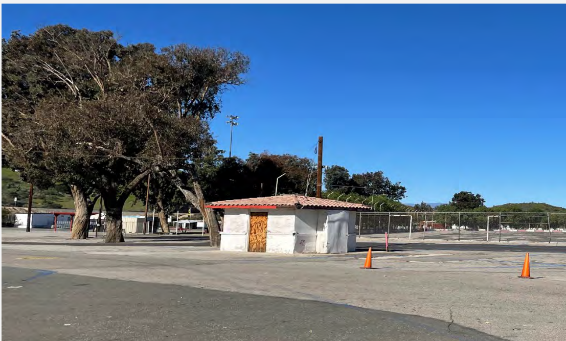
Figure 13. Overview of one of the six identical Concession Stands (6), view looking north (IMG_2200).
