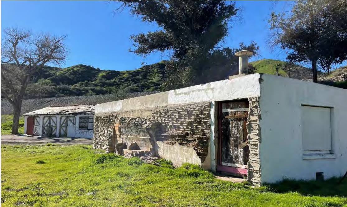
Figure 6. Overview of Baker Residence (1) showing main (east) and north elevations. Looking southwest (IMG_2296).
