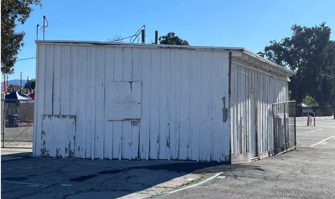
Figure 10. Oblique of Ancillary Building's (4) primary (southwest) and side elevations. View looking east (IMG_3171).
