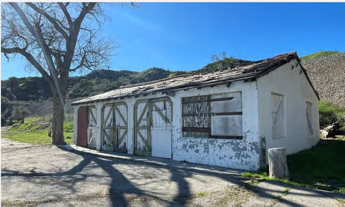
Figure 7. Overview of the Stable (2) showing primary (east) and north elevations. View looking west (IMG_3272).
