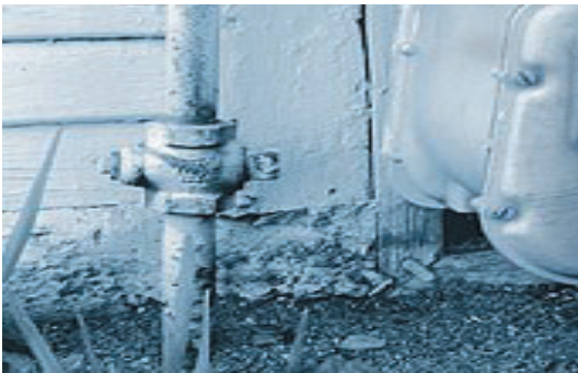
Gas On /Off valve
