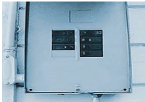
Electric Breaker Panel
