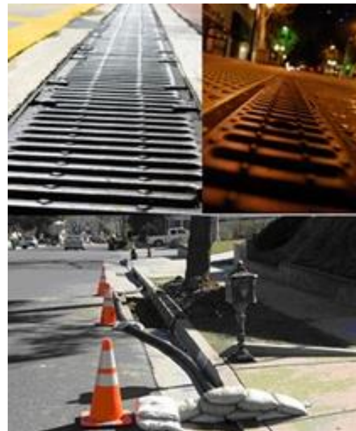
Figure 45: Storm Drain Debris Mitigation
