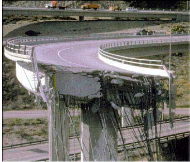
Figure 27: Freeway Collapsed Interchange
