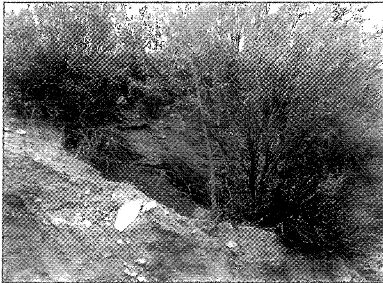
Drainage B – View of leaking pipe and 4' x 4' created wetland near drop structure
